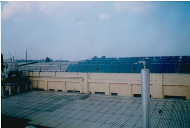
Solar Water Heating System at Leo Leather Industry Jullundhar
