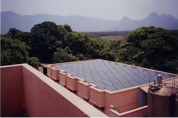
Solar Water Heating System at MILMA Dairy
