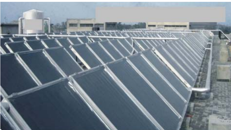
12 Lakh Kcal per day system for Nickle Bath at Kangaroo Industry Ludhiana
