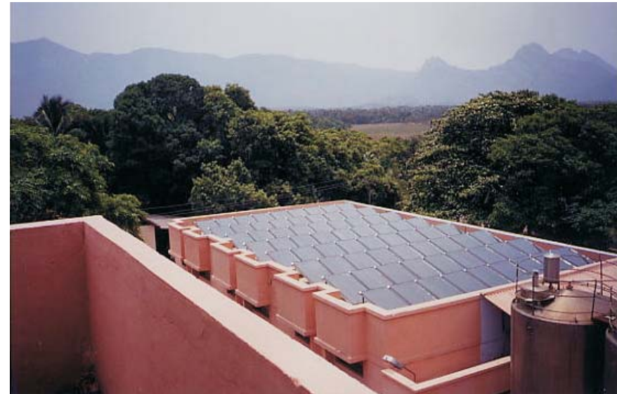
Solar water heating system at the MILMA Dairy, Kerala
